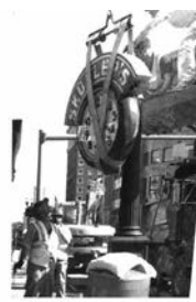
As part of Main Street construction, workers remove the clock face from its column. Fabricating commenced and the clock made its way to Cincinnati for restoration. (City of Lexington Historic Preservation Office, 2010)
