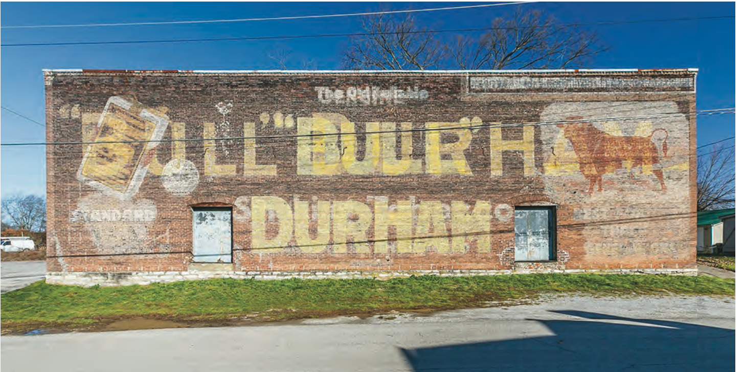
Tobacco warehouse in Georgetown, Scott County. Blocks away from Georgetown College and the downtown commercial district. Great opportunity for adaptive reuse!
