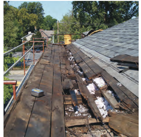
Wooden base under an old box gutter
