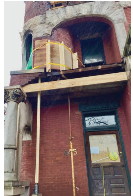
In order to rebuild the base of the turret, the upper portion had to be belted to the house.
