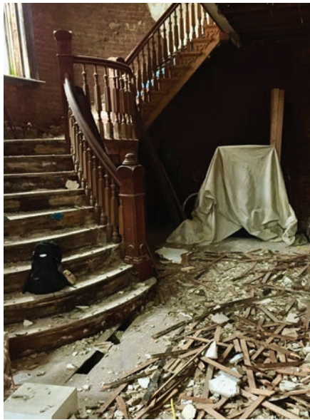
Molded and rotten wood had to be removed before renovations could begin. The entire project extended for over 16 months.
