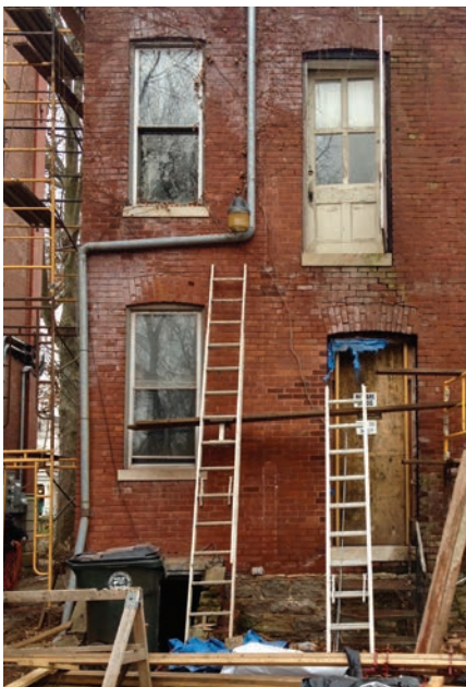
The back porch had fallen off the house leaving a second floor door going to nowhere.
