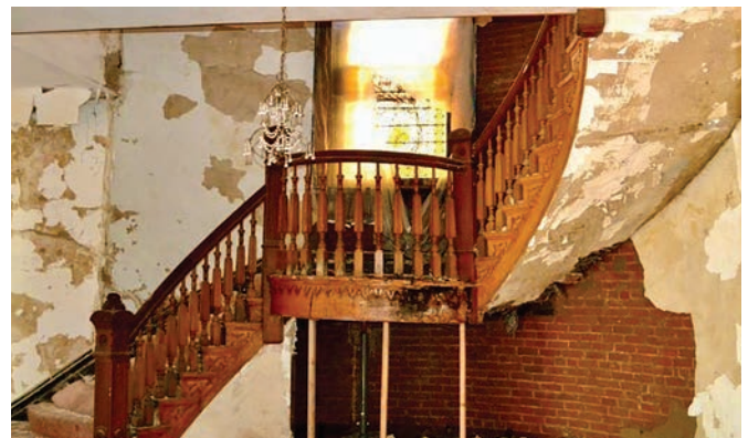
Two views of the circular staircase before renovations began. Notice the hole in the floor where the wood had rotted through.
